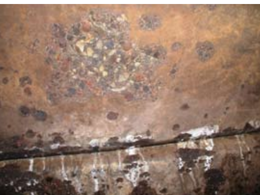
(Photo-Top) A blazing car fire caused damage to a bridge in Washington County, Ore., but the effects were minimal and the bridge was reopened to traffic after an inspection.
