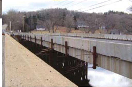
A temporary bridge in Connecticut made use of precast concrete adjacent box beams that had been stored for more than 10 years after earlier use for another temporary bridge.
