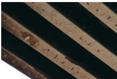
The heat from the Puyallup bridge fire was intense enough to cause some spalling, which left some exposed strands, but it left them undamaged.
