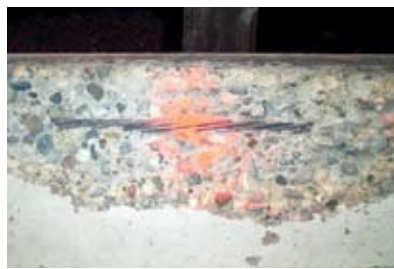
The pink color shown in this girder from the Puyallup bridge fire indicates that the concrete was exposed to temperatures higher than 500 °F.
